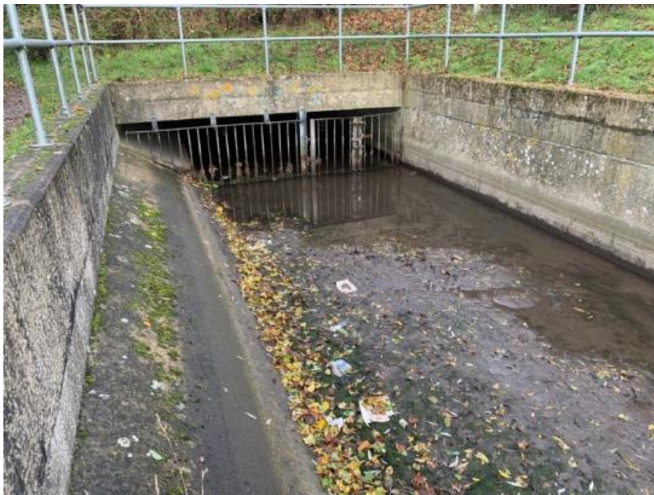
Figure 6.2: A channelised section of the Upper Duke of Northumberland’s river at the entrance to a box culvert, reflective of conditions across large sections of the river. Concrete bed and banks, low water levels, with no presence of aquatic macrophytes or quality habitat and only a small covering of moss, algae and leaf litter.
