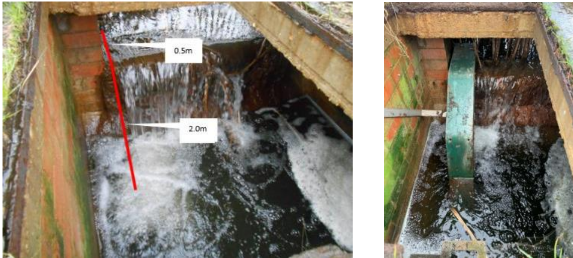
Figure A1.2: Before (left) and after (right) images of an eel pass installed to the sump of the off-take of Rick Pond.
