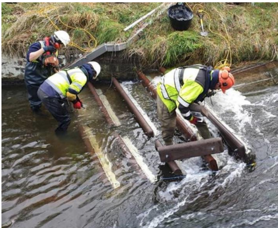
Figure 4.3: Image of improvement works (fish pass installation) being carried out by FishTek at Mogden Barrier 3.
