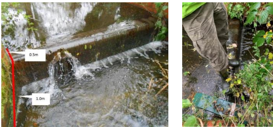
Figure A1.3: Before (left) and after (right) images of an eel pass installation to a vertical weir in Home Park.
