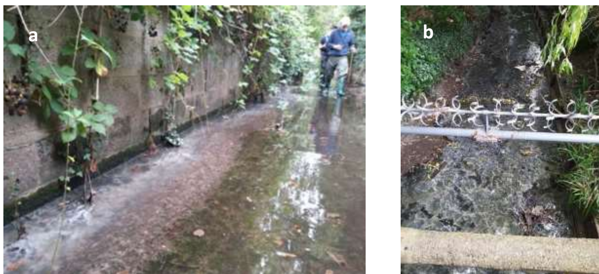
Figure 16: Photos of (a), Thistledene Avenue, upstream of the culvert, and (b), Field End, Ruislip, during the 2021 Outfall Safari showing extensive sewage fungus covering the riverbed.
