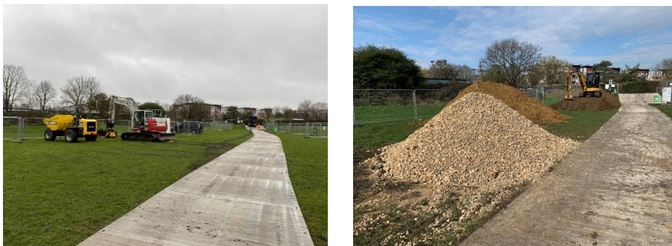
Figure 4.2: Temporary road and construction site built for the duration of the restoration project. Left image credit: ©Wild Future.
